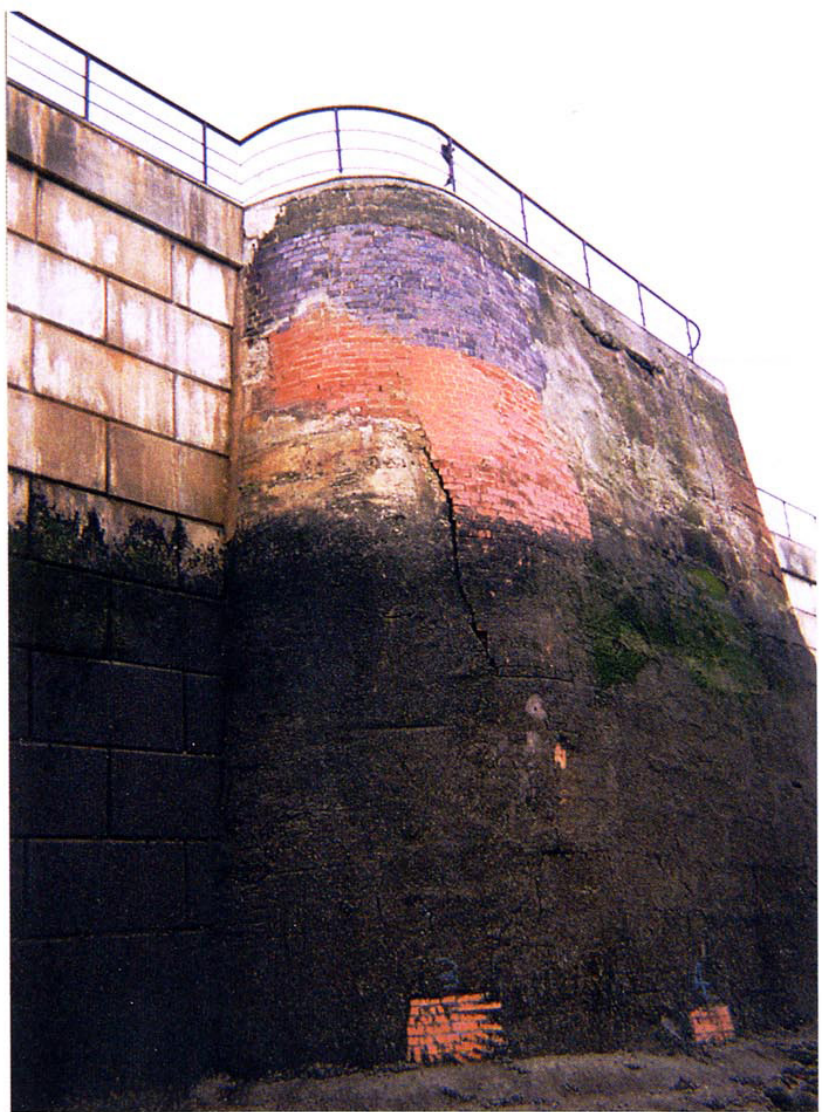
Figure 3: Previously repaired area
